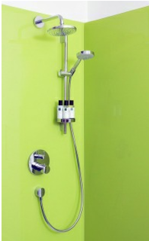
Shower Room Fitted with Easy Glass Splashbacks Bespoke Lime Green Shower Wall Panels
