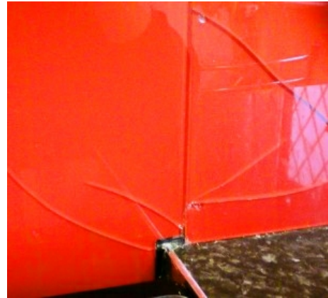
Photograph showing how untoughened glass splashbacks crack when damaged
